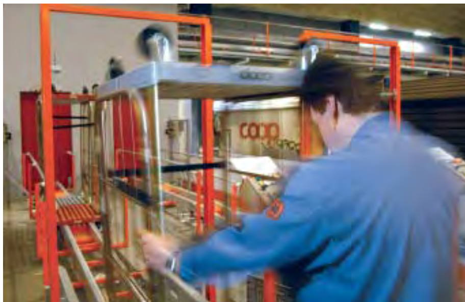
Thanks to Rapid Link, the operating personnel can shut down segments of the conveyor at all times and immediately remedy faults.
